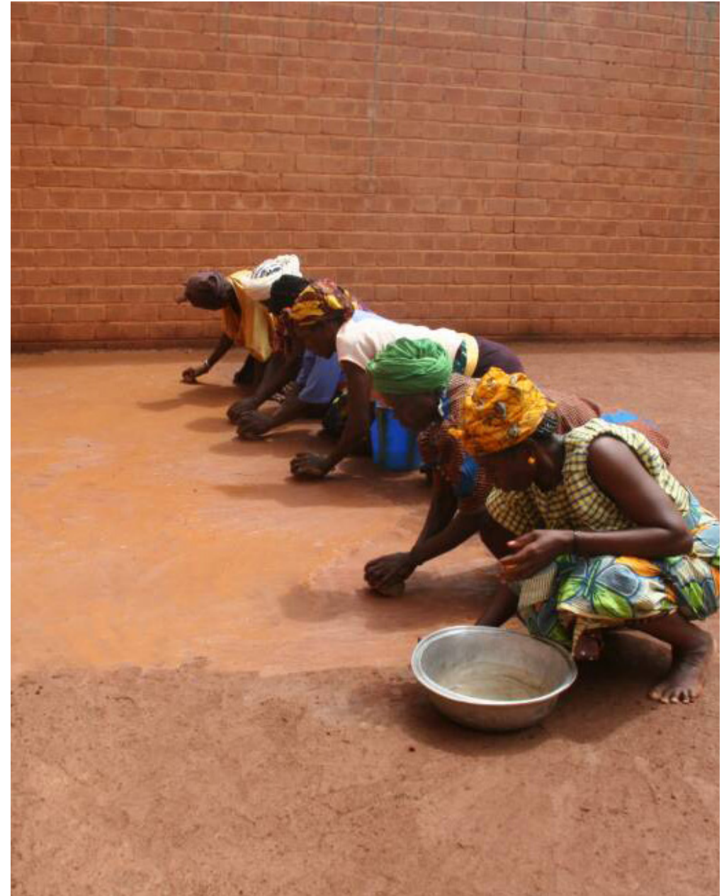
Figure 7, Kéré Architects, 2008. Community members flattening the floor during the construction of the Gando Primary School Extension. [Photograph]
